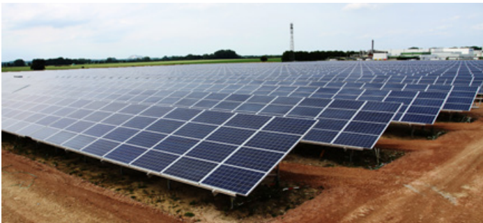
Image 1: Panel strings in a utility installation
